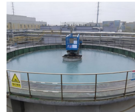
Physicochemical Sedimentation Tank
