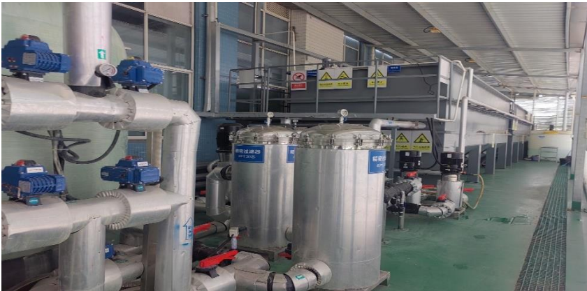
Upgraded treatment system with improved wastewater reuse rate
