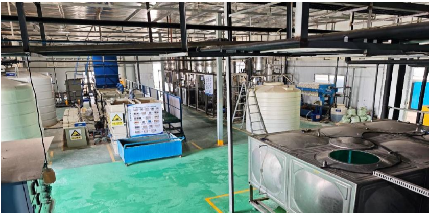
New treatment system for wastewater from de-welding and grinding cleaning processes
