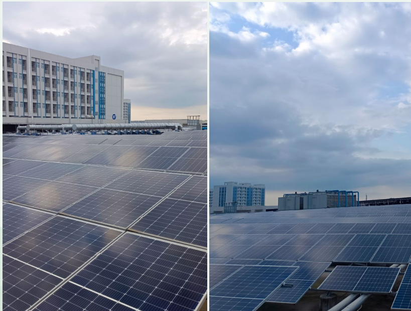
Rooftop PV Panels Installed in Jiangxi Park
