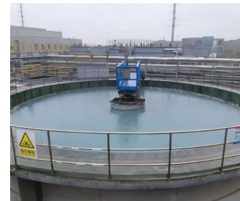
Physicochemical Sedimentation Tank
