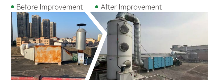
Huarong Communication Waste Gas Treatment Facilities and Process Upgrades
