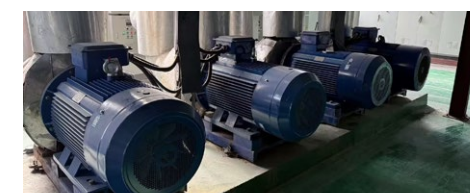
Luxcase ICT Yancheng Energy-Saving Motor Replacement
